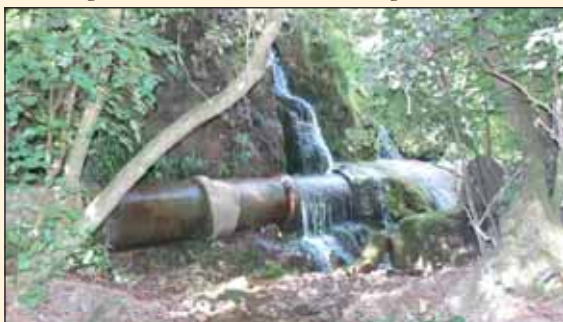
Old Penstock Pipes, Maraetotara
